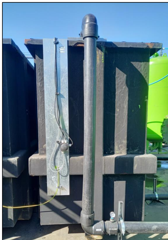
Figure 13. Backwash tank T5
