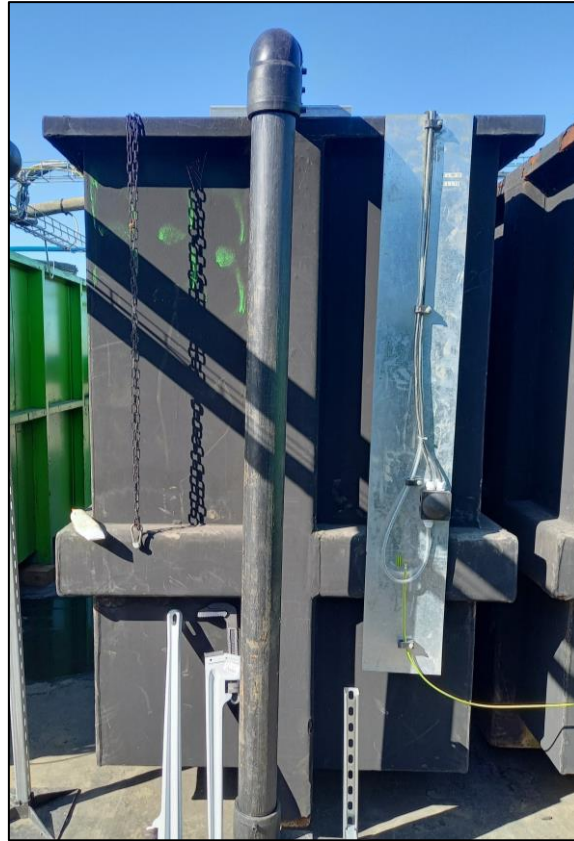
Figure 12. Backwash tank T4
