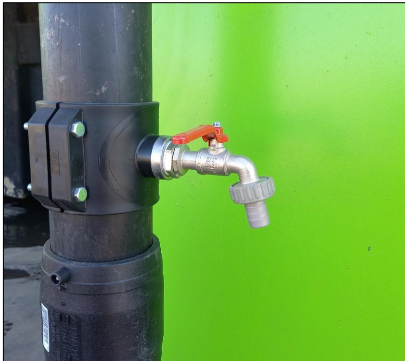
Figure 11. Sample tap at system inlet (T1)
